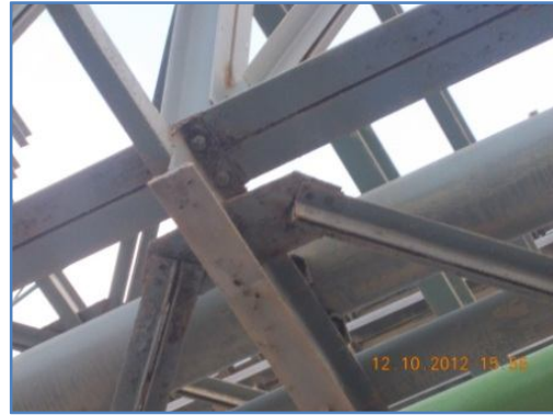
Nut bolts missing on cross bracings
