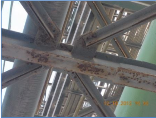
Corrosion and scaling
