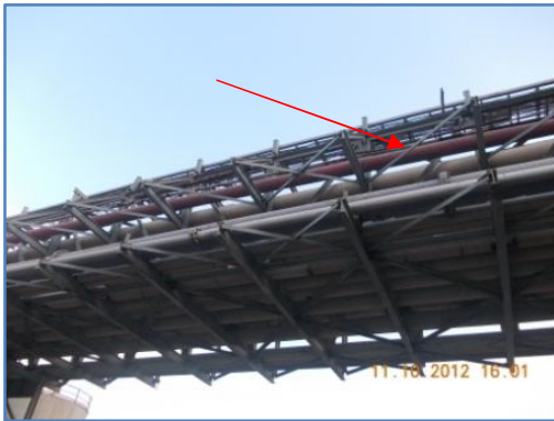
Cross bracing missing
