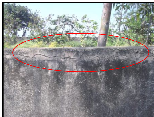
Cracks noted on the R.C.C dyke wall.
