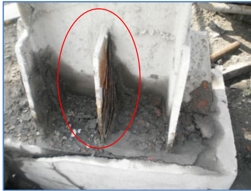
Severe corrosion and scaling
